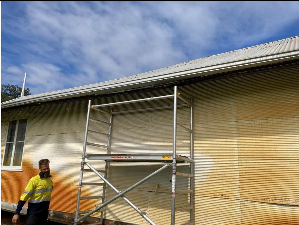
Photo 13: Scaffold set up and inspection access point on the Northern end of the croquet clubhouse.
