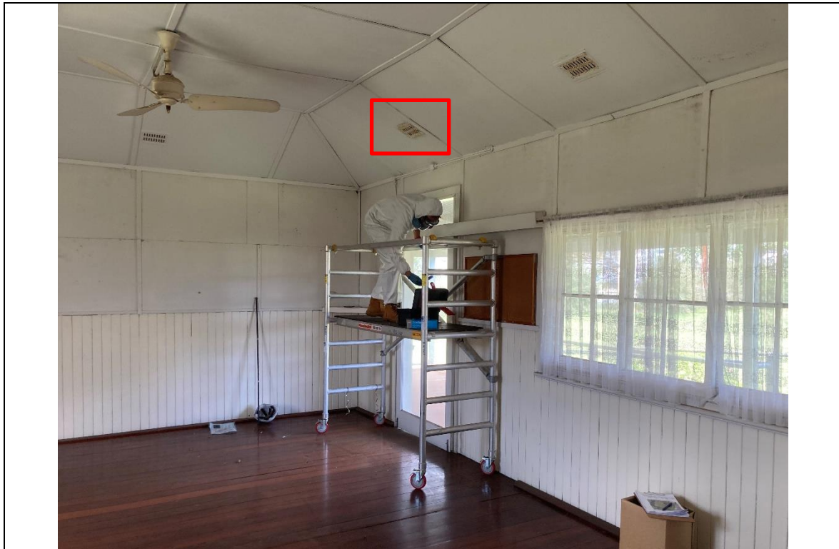
Photo 31: Set up the platform and carried out roof inspection through the air vent. Inspectors were well-protected from asbestos by wearing the proper PPE.
