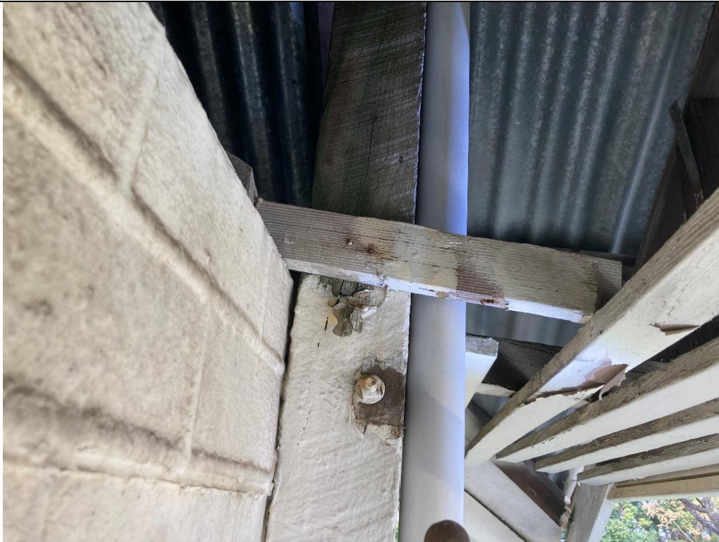
Photo 9: View of the bolt connection to purlin prop.
