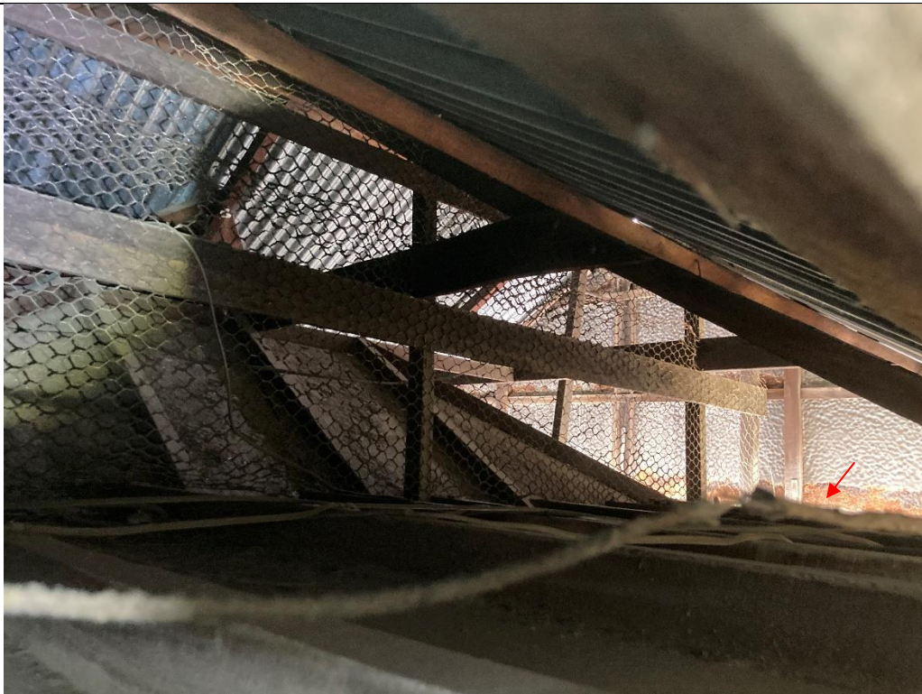
Photo 14: Overall view of the roof condition. Widespread corrosion on the internal cladding.
