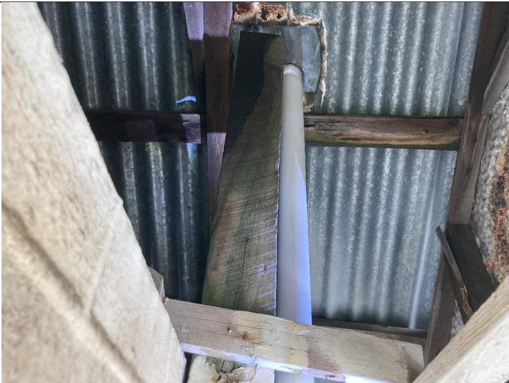
Photo 8: View of purlin prop and localised corrosion on roof sheet.
