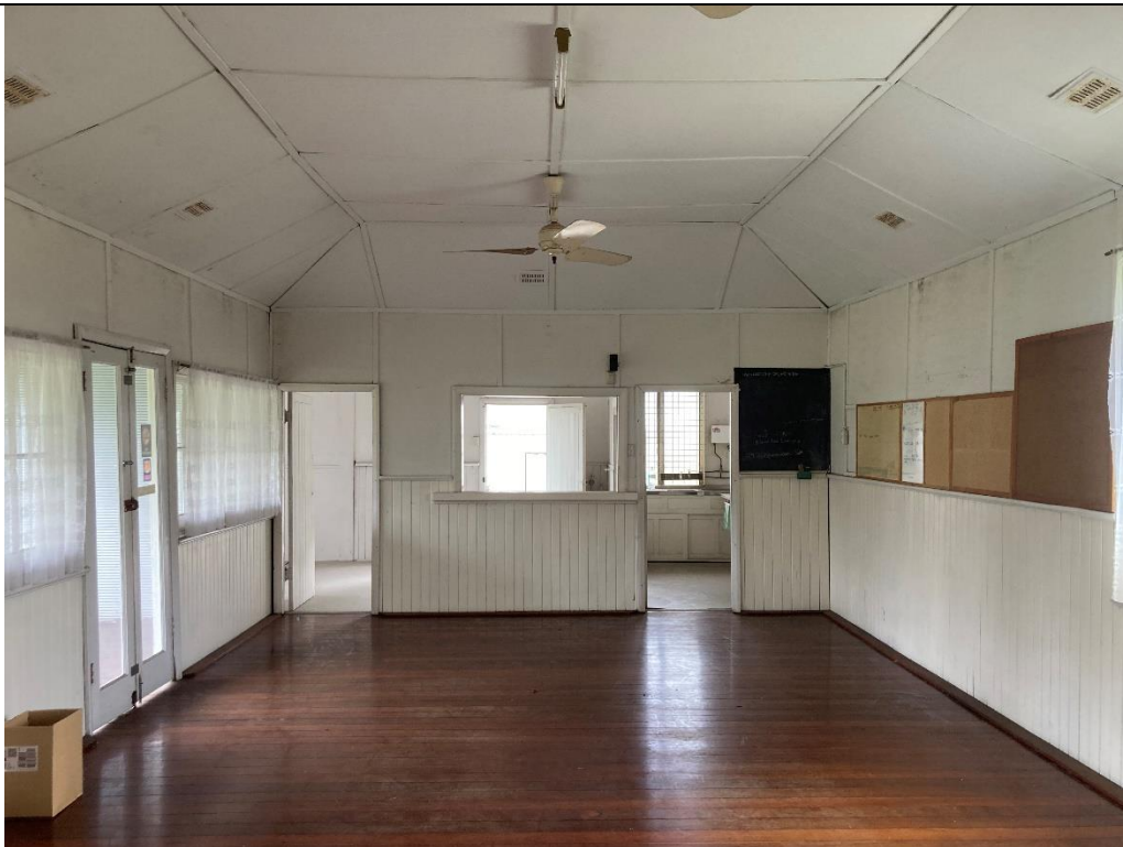
Photo 29: Interior view, looking West. Observed Asbestos fibre cement sheeting product at the internal wall.
