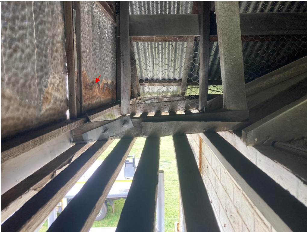
Photo 6: View of the wall plate connection and timber eaves on the West side. Widespread corrosion on the internal cladding.
