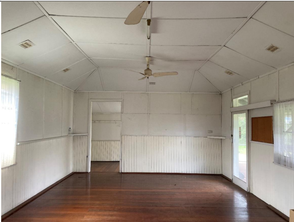
Photo 30: Interior view, looking East. Observed Asbestos fibre cement sheeting product at the internal wall.
