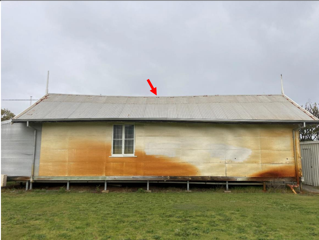
Photo 2: Overall view from the North of the croquet clubhouse looking South. Observed sagging of the roof ridge beam.
