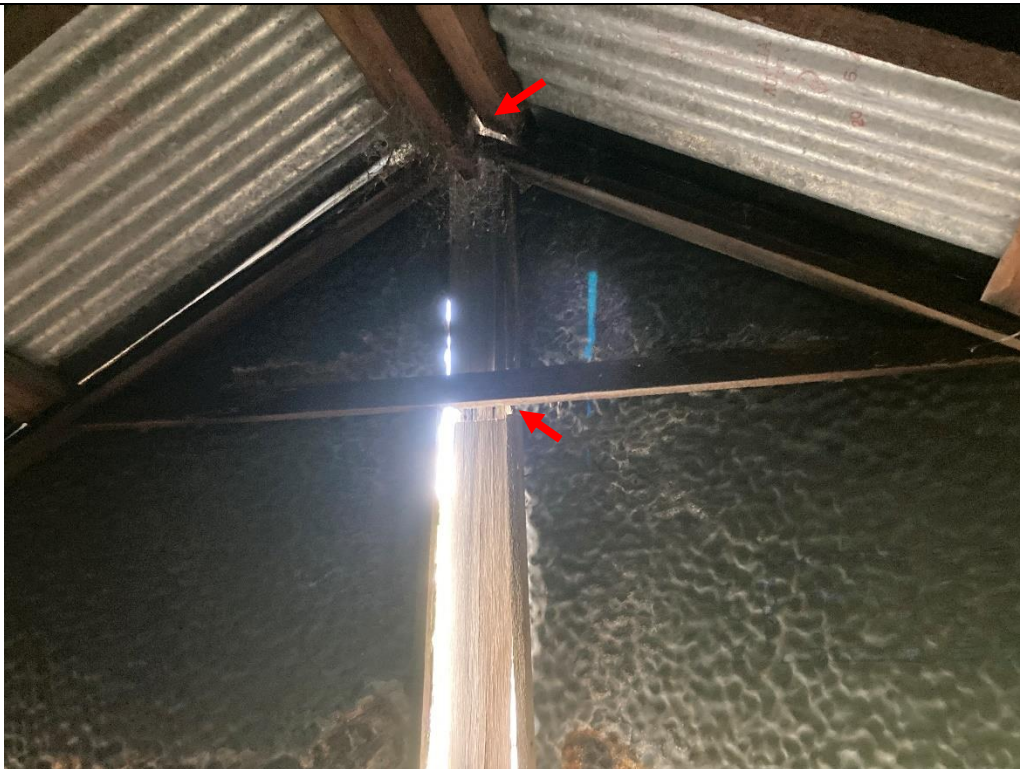
Photo 33: Observed skylight and timber split.
