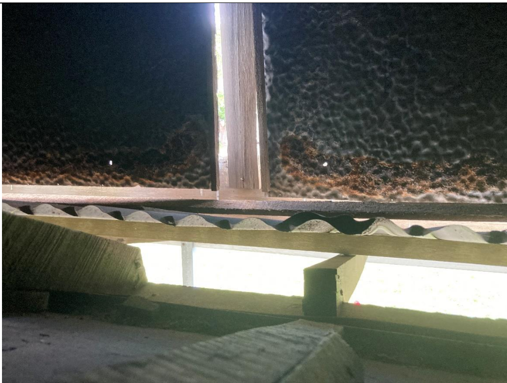
Photo 34: View of the stud and top plate. Localised corrosion on cladding sheet.
