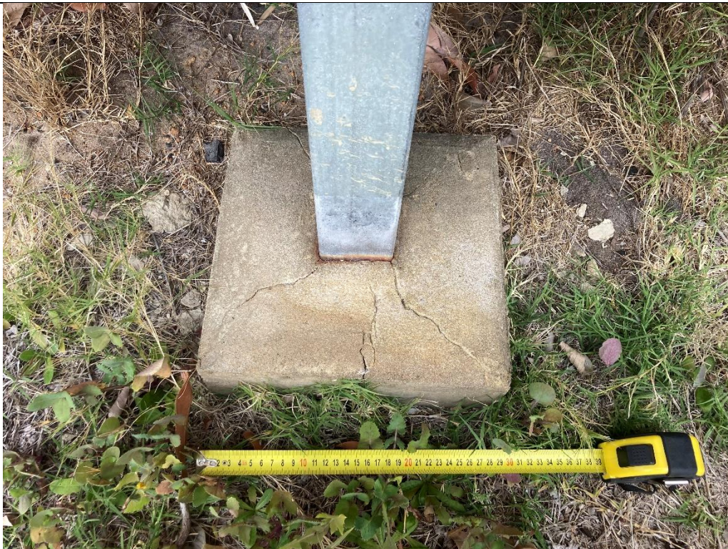
Photo 10: Observed cracks on the pad footing.
