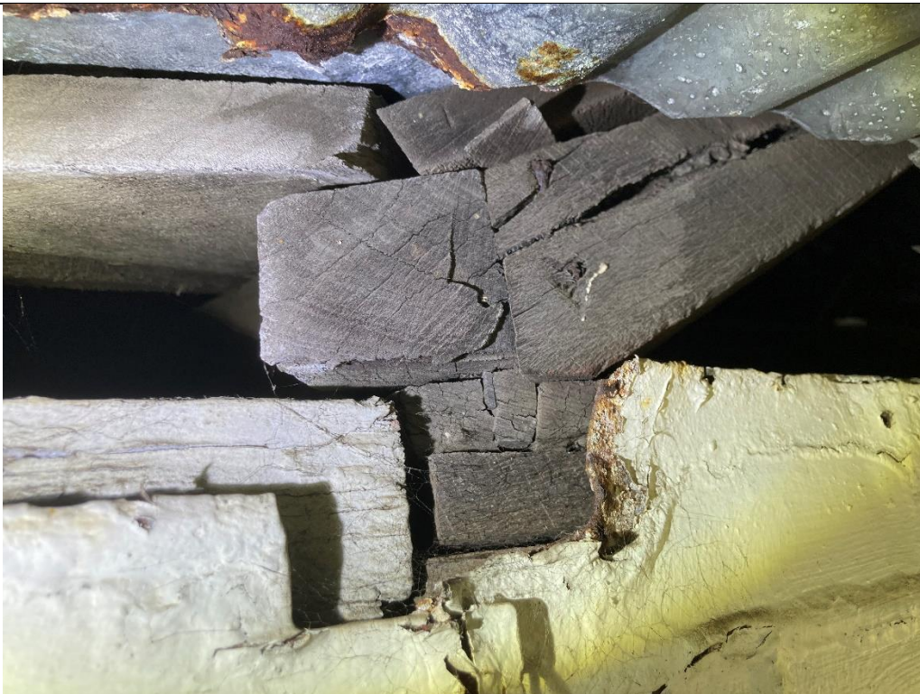
Photo 26: Observed timber splits on the top plate, refer to Photo 23.
