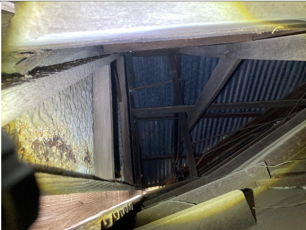
Photo 22: View of rafter beam, vertical posts and rafters, from North to South.
