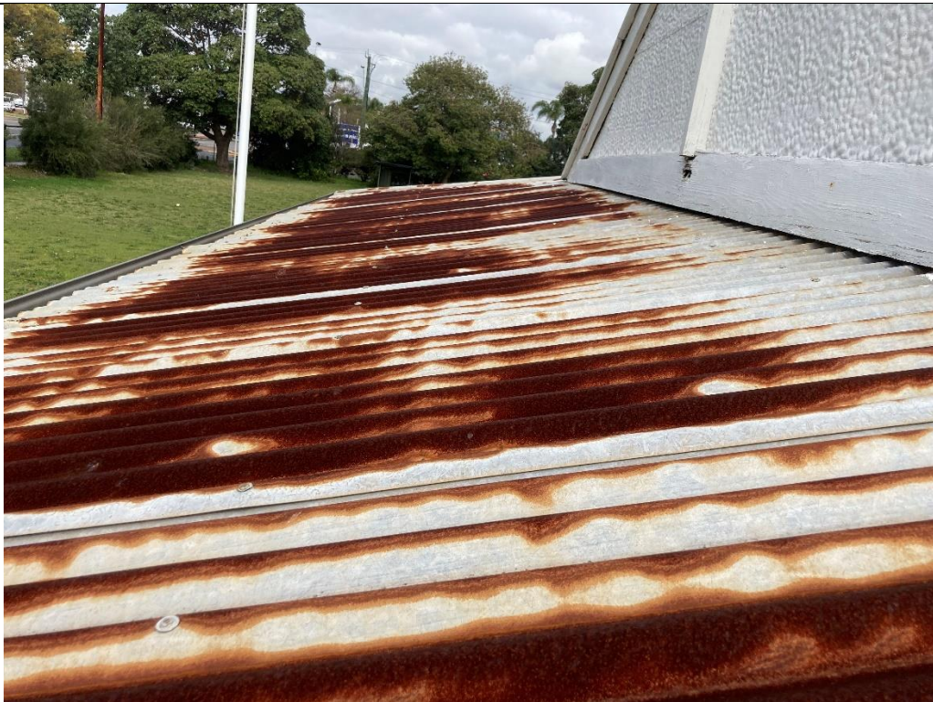
Photo 20: View of the corrugated roof sheet, looking South – showing significant corrosion and rust.
