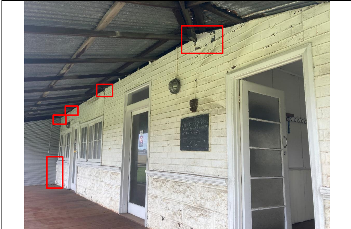
Photo 23: Overall view of the South side of the croquet clubhouse showing localised deformation on the cladding.
