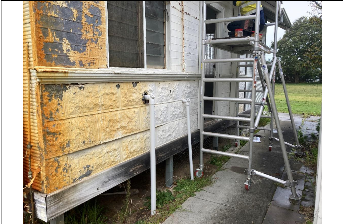
Photo 3: Scaffold set up and inspection access point on the Western end of the croquet clubhouse.
