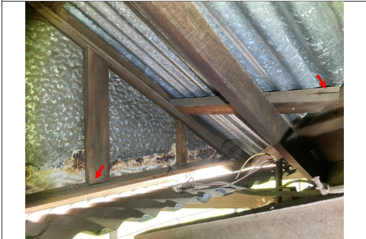
Photo 32: Observed timber splits at nail connections.
