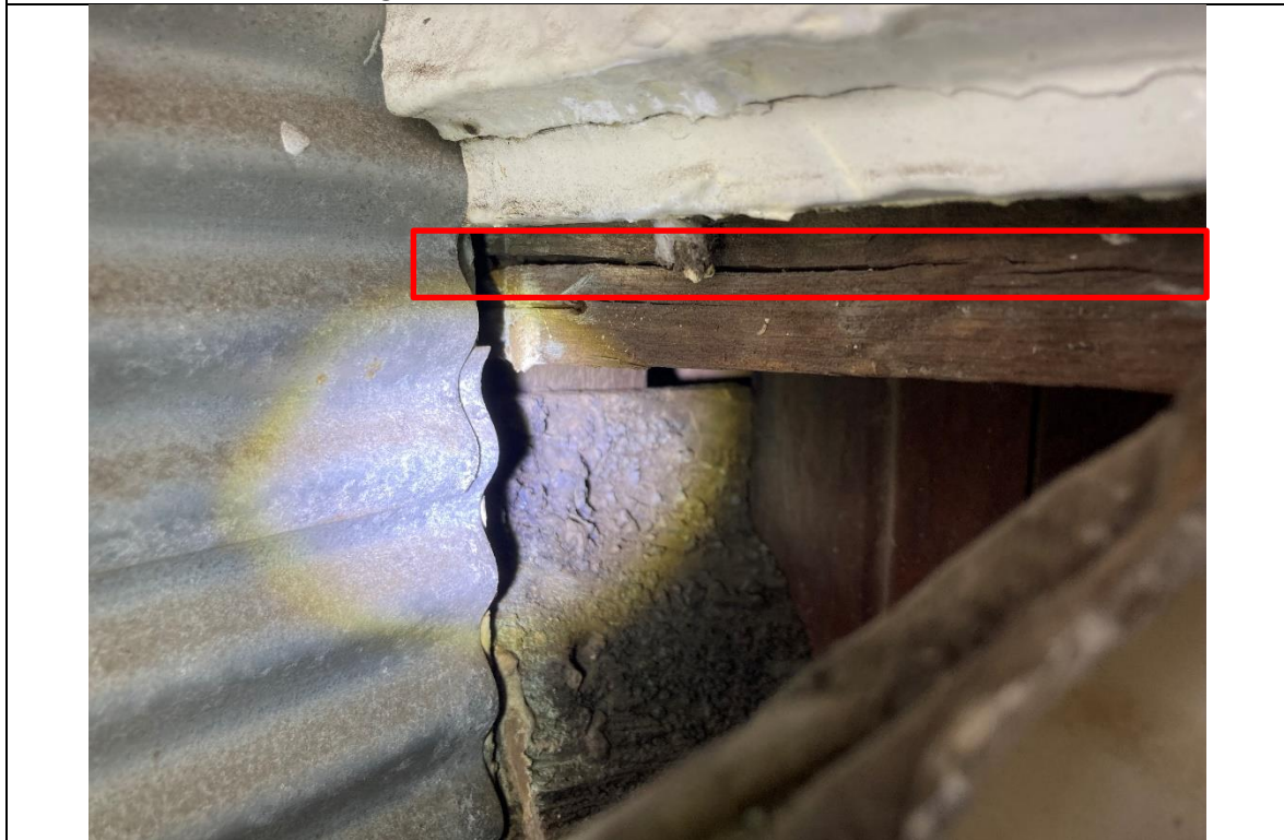
Photo 24: Transverse crack (refer to Photo 23).
