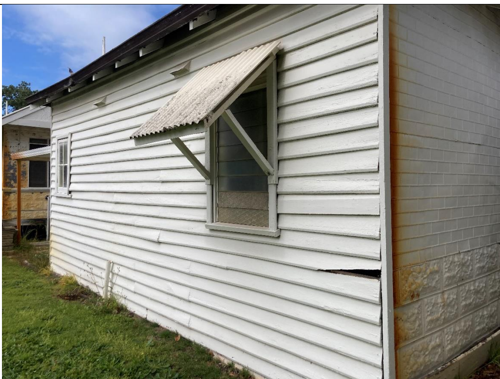
Photo 40: Overall view of the cottage, looking South. Corrosion and rust stains on wall cladding.
