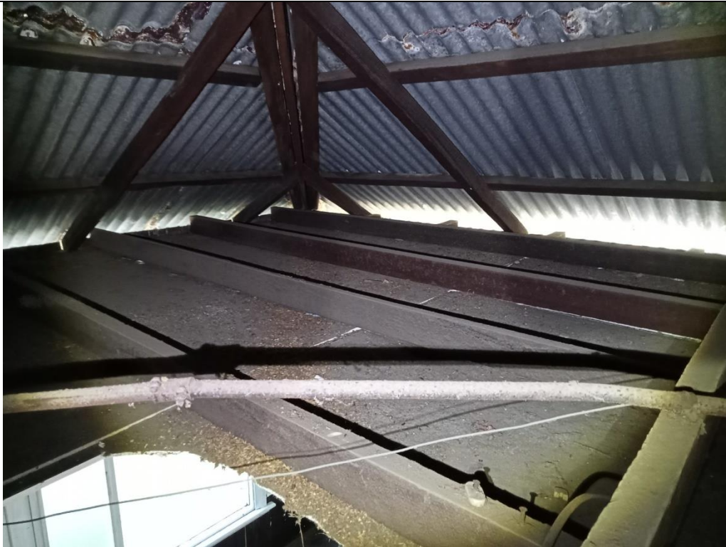
Photo 43: Overall view of the ceiling and rafters. Roofing sheets showing corrosion.
