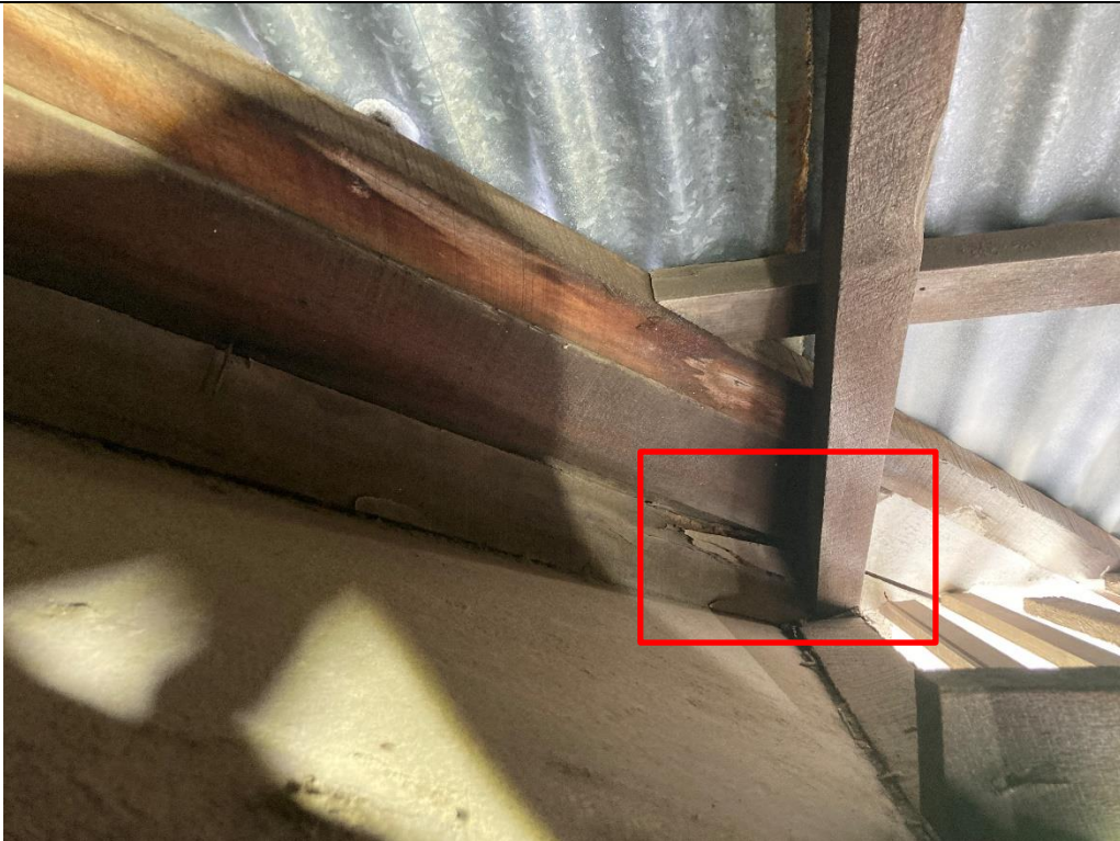
Photo 7: View of the rafter and beam connection – showing localised timber splitting.
