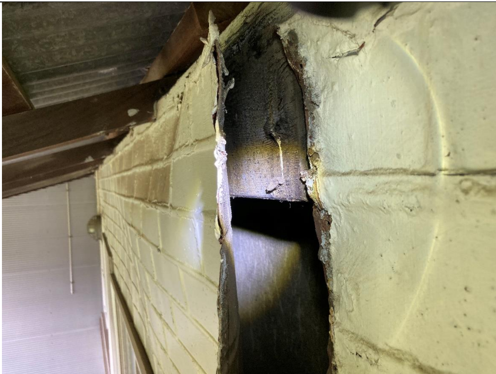
Photo 28: Delaminated cladding to wall frame, refer to Photo 23.
