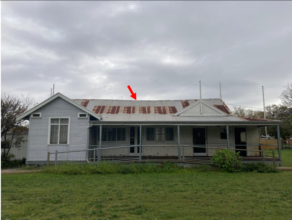
Photo 1: Overall view from the South of the croquet clubhouse looking North. Observed sagging of the roof ridge beam.
