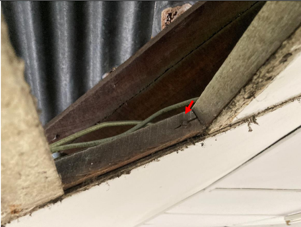
Photo 37: Observed timber split at nail connection of the ceiling joist.
