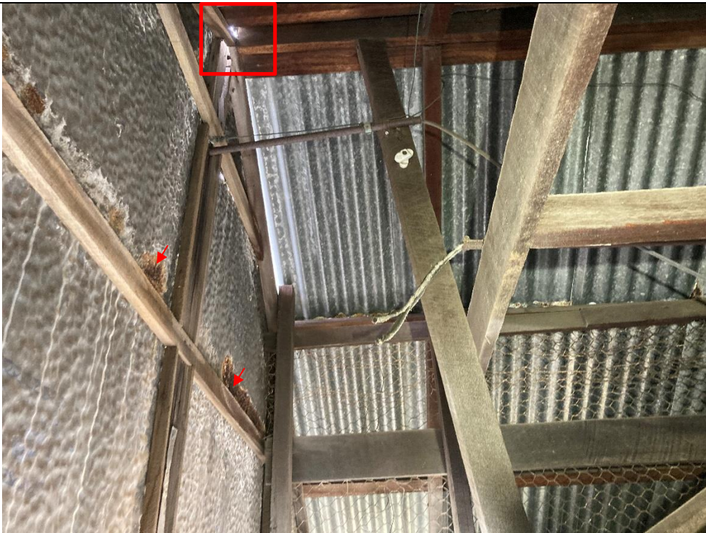
Photo 5: Skylight at purlin prop to beam rafter connection. Widespread corrosion on the internal cladding.
