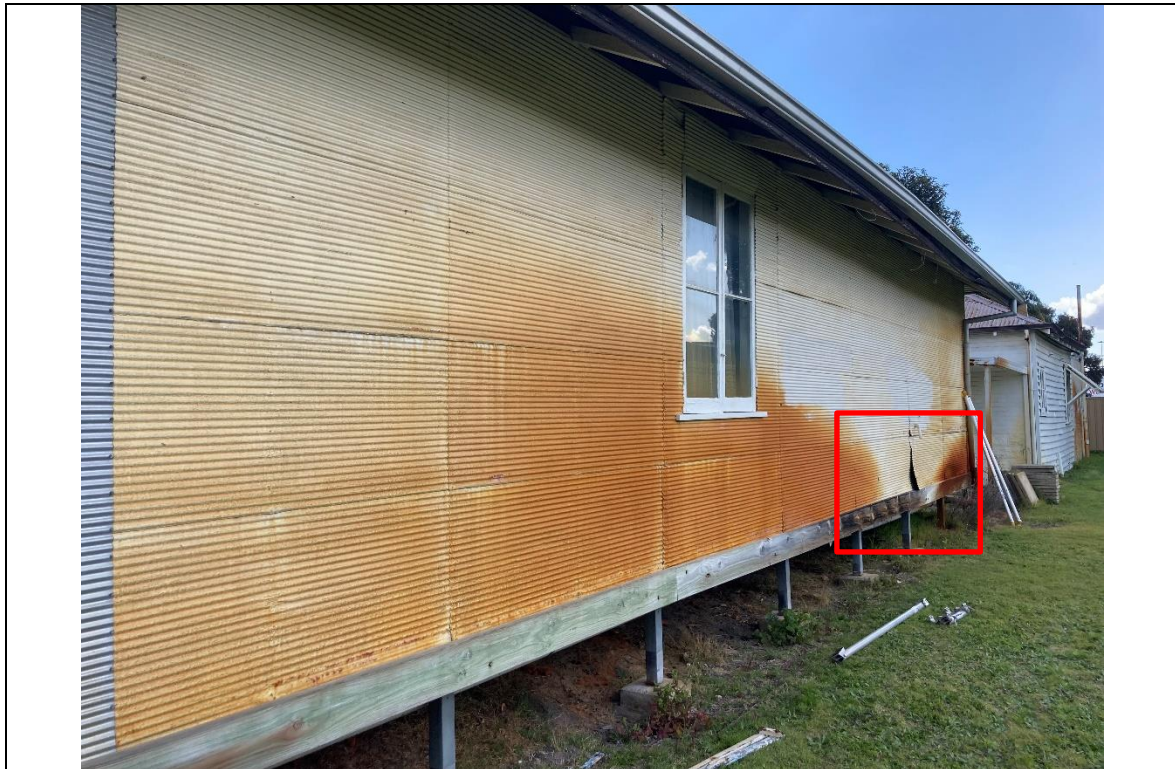
Photo 17: Overall view of cladding on the Northern end of the building – showing significant corrosion stains and localised defect.
